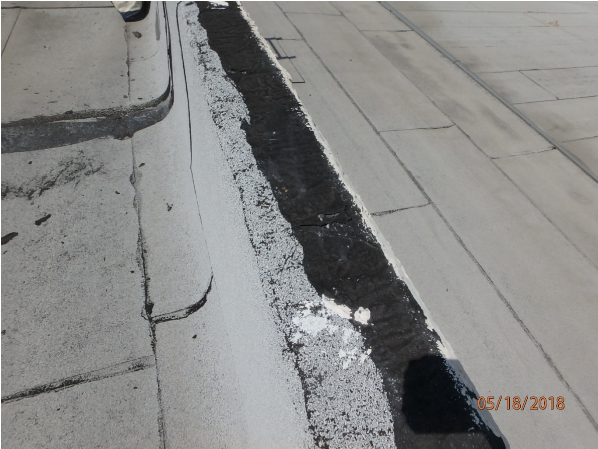
Prep, apply reinforcement fabric and coating to the tops of the existing parapet walls
