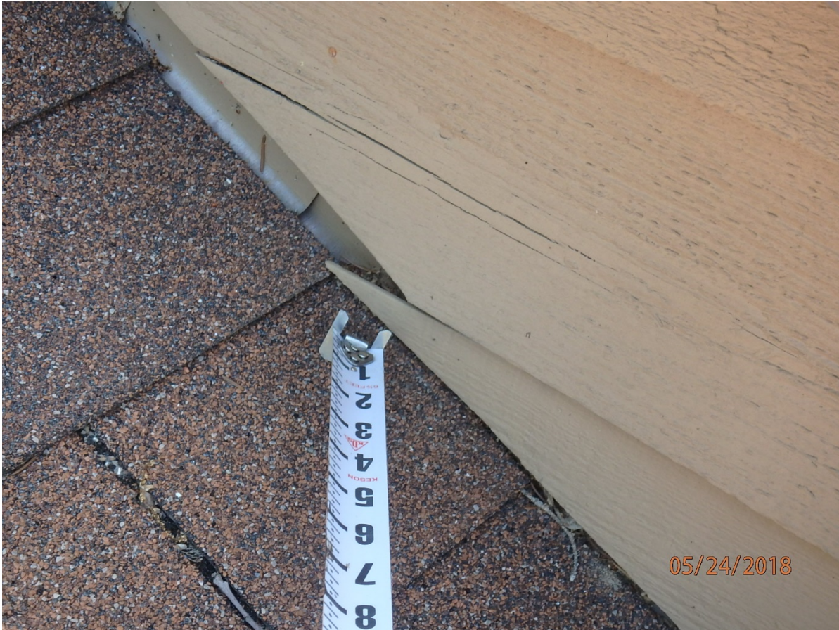
Replace all broken or damage siding at roof to wall
