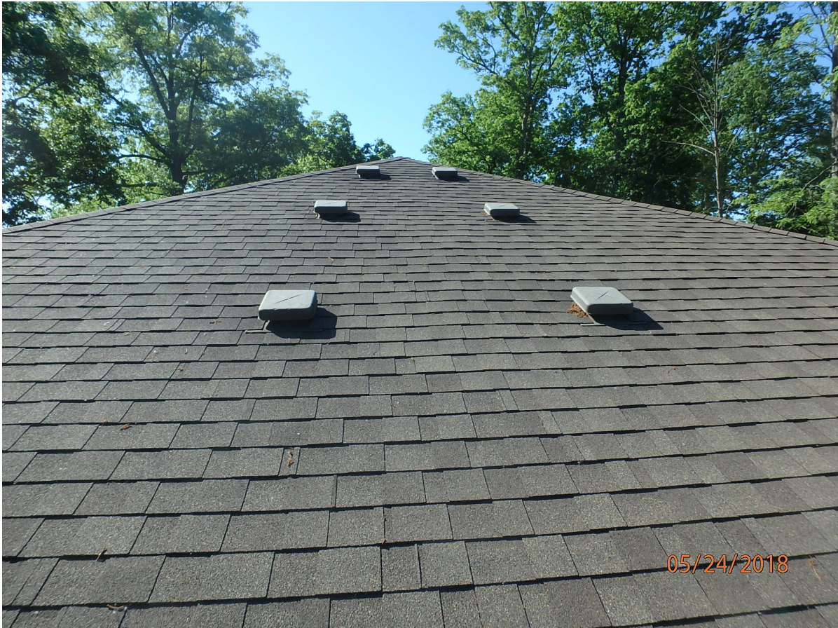
Reuse static vents if can be salvaged / Clean, prime and paint to match Shingles
