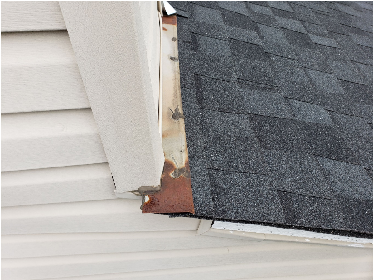
Replace rusted head wall flashing
