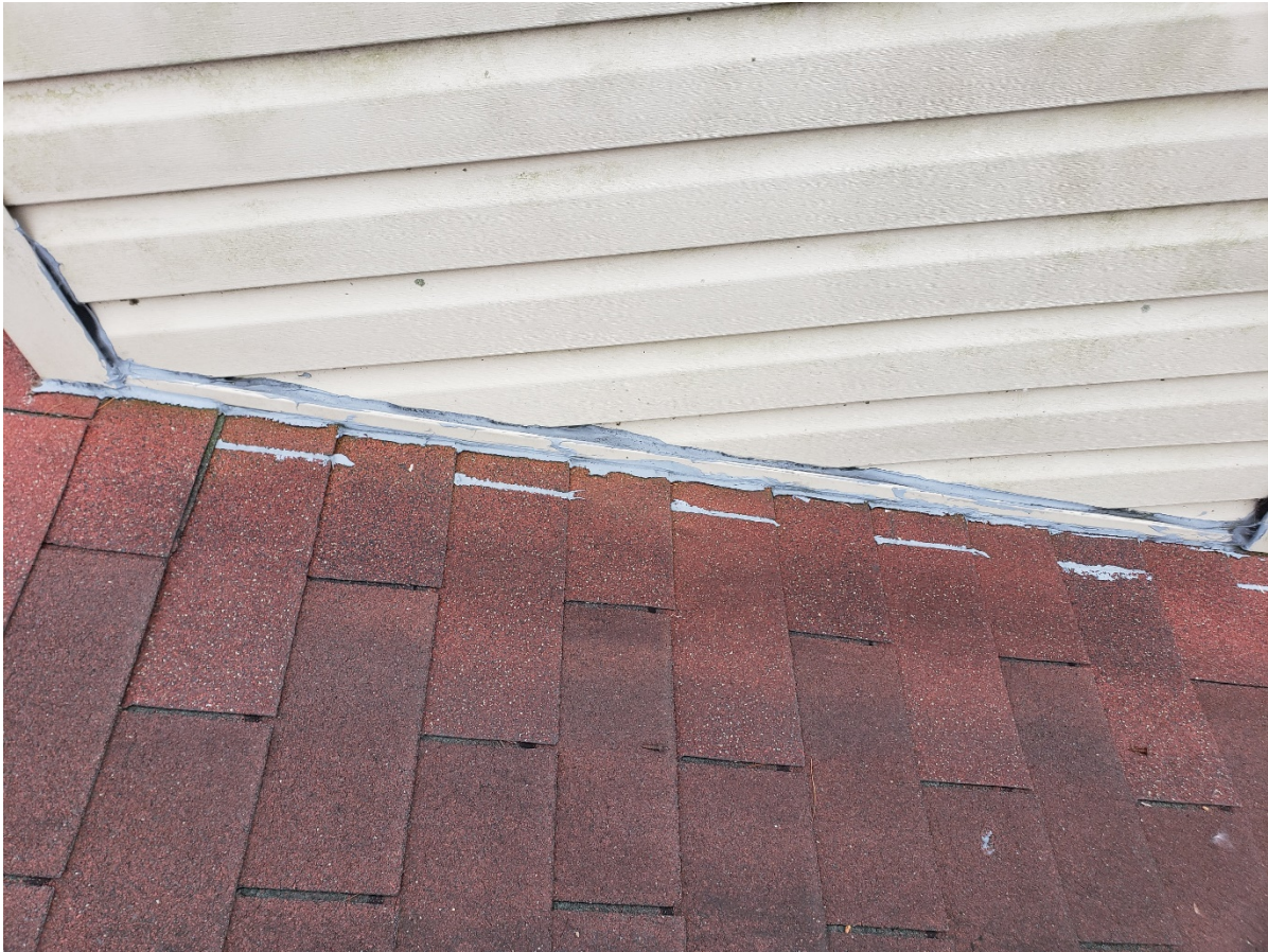
Remove siding to install new step-flashing and raise 1-1/2 to 2 inches above roof
