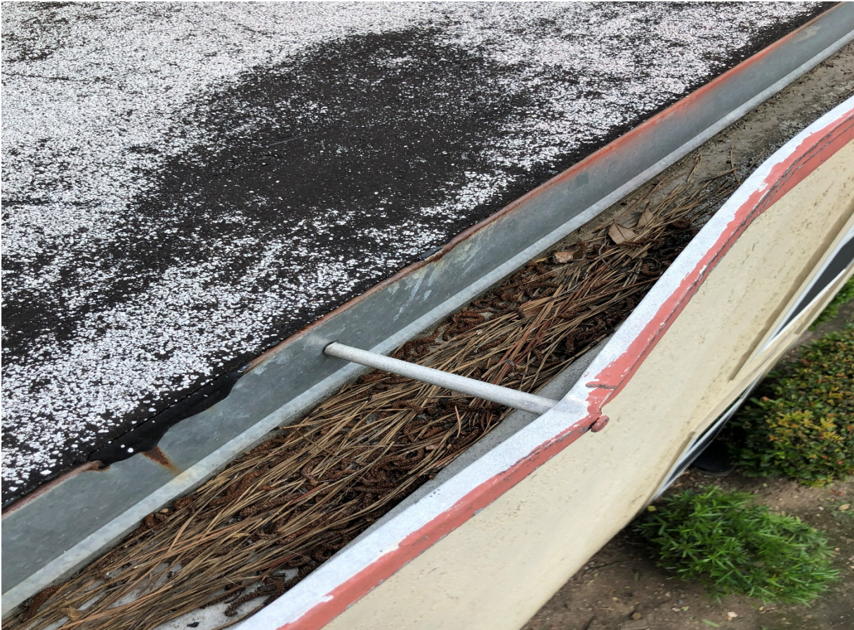
Replace bent or damaged gutters
