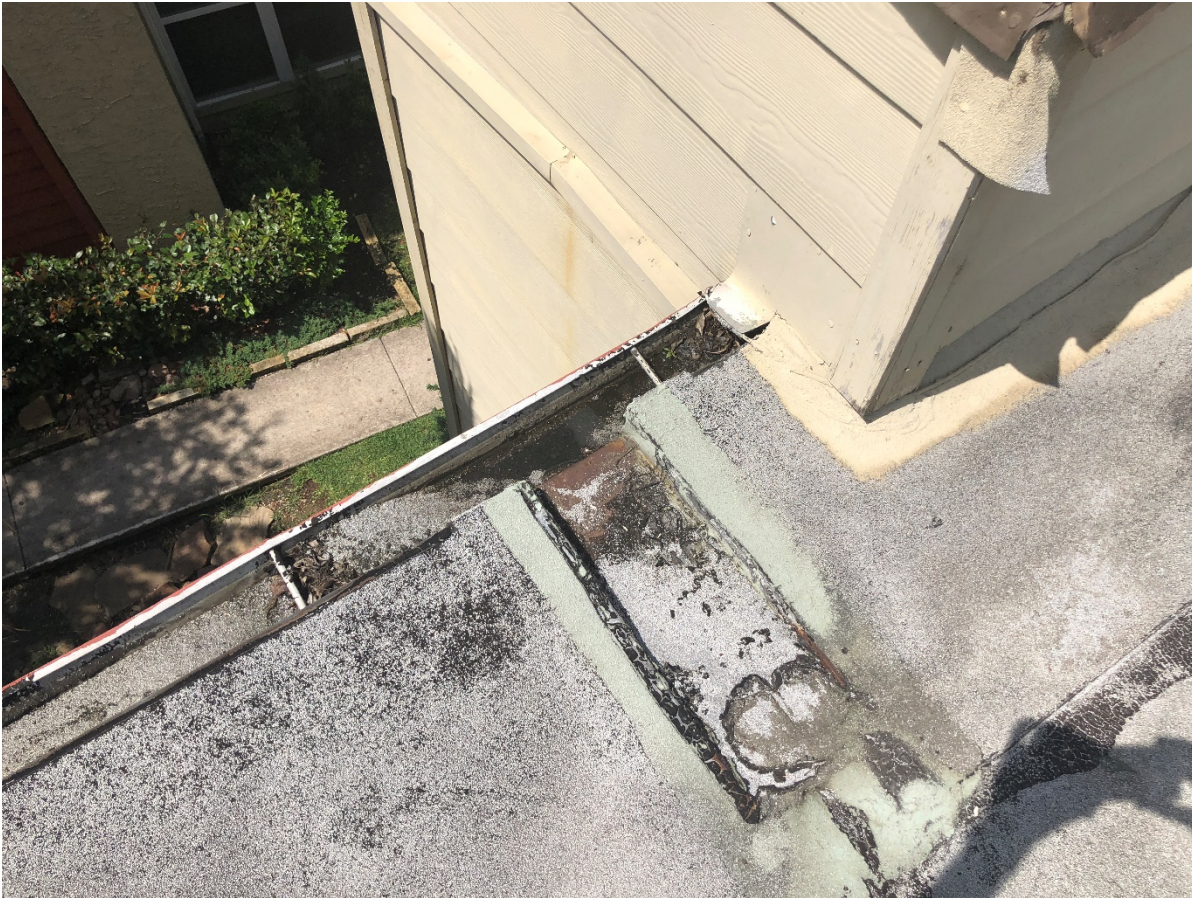
New scuppers for the reroofing and clean and patch scuppers for repairs
