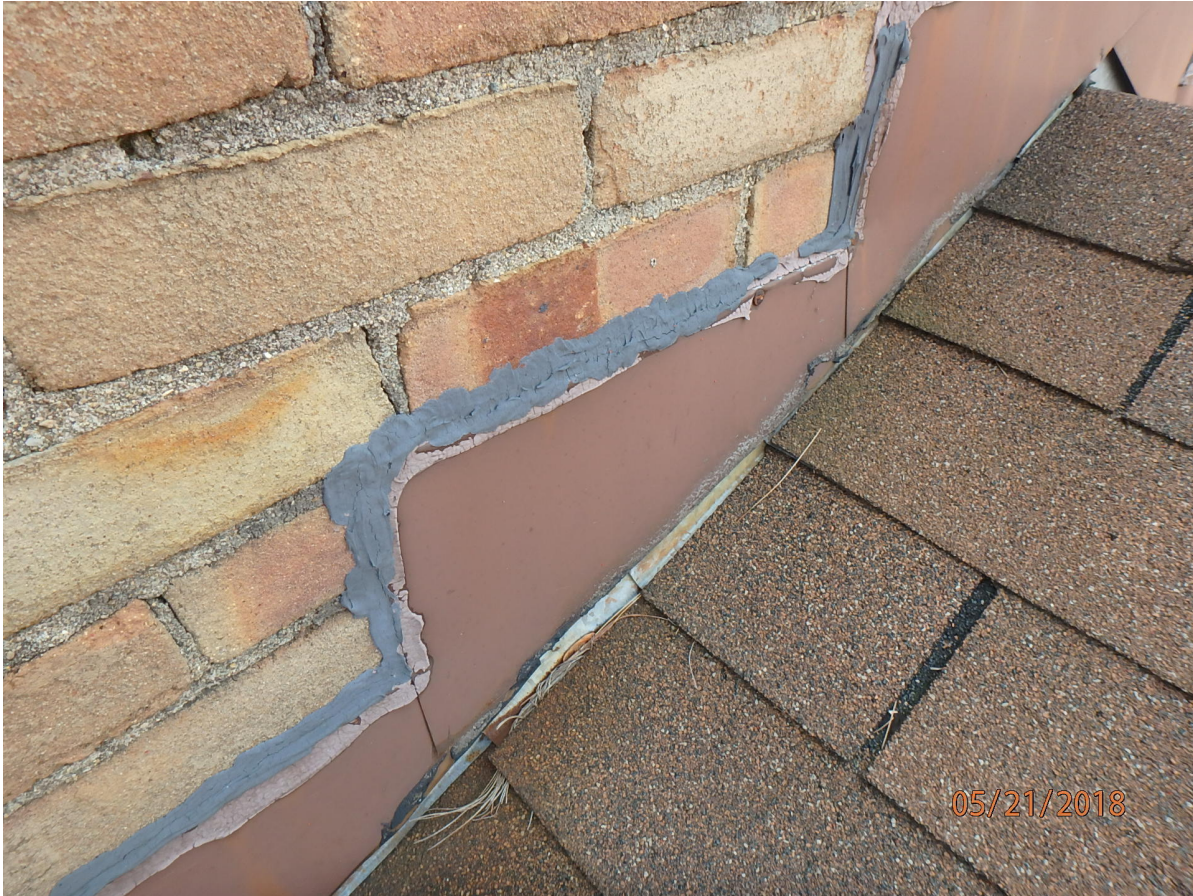
Remove and install new step flashing / Clean ALL old sealant from counterflashing and install new Counter-flashing per NRCA guide lines
