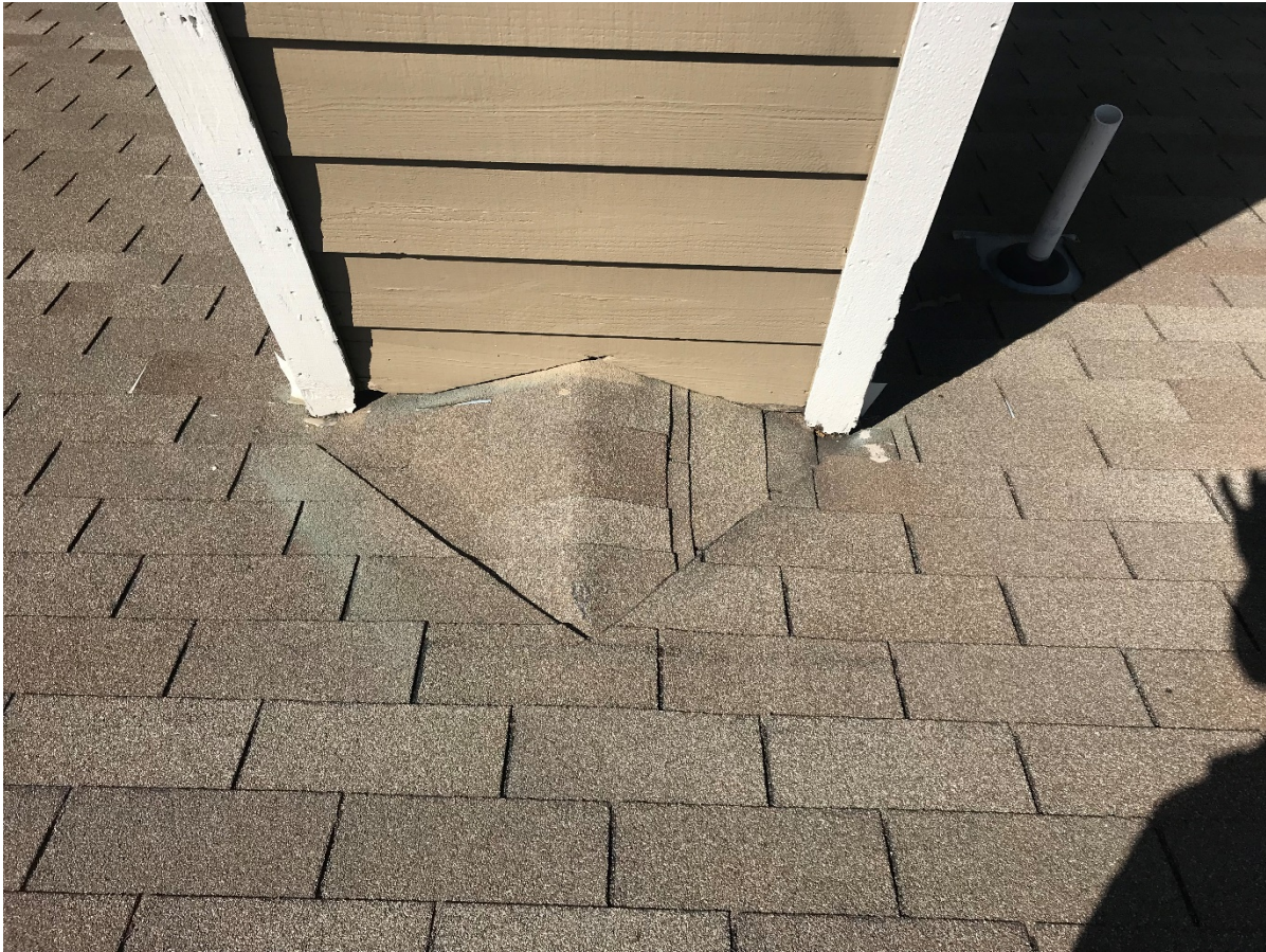
Remove siding to install new step-flashing and raise 1-1/2 to 2 inches above roof, on all three sides
