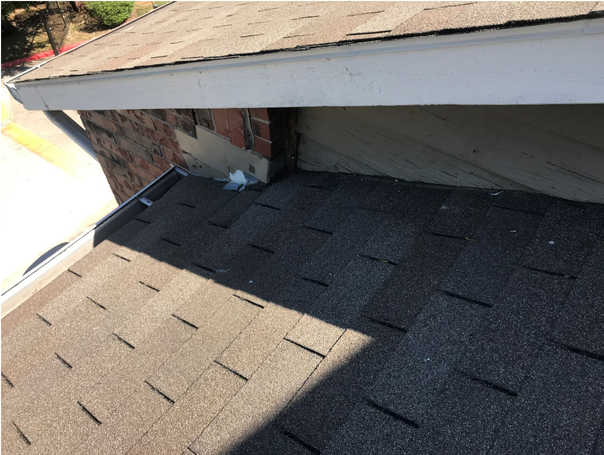
Add in cant at corner of brick to wood siding to divert water
