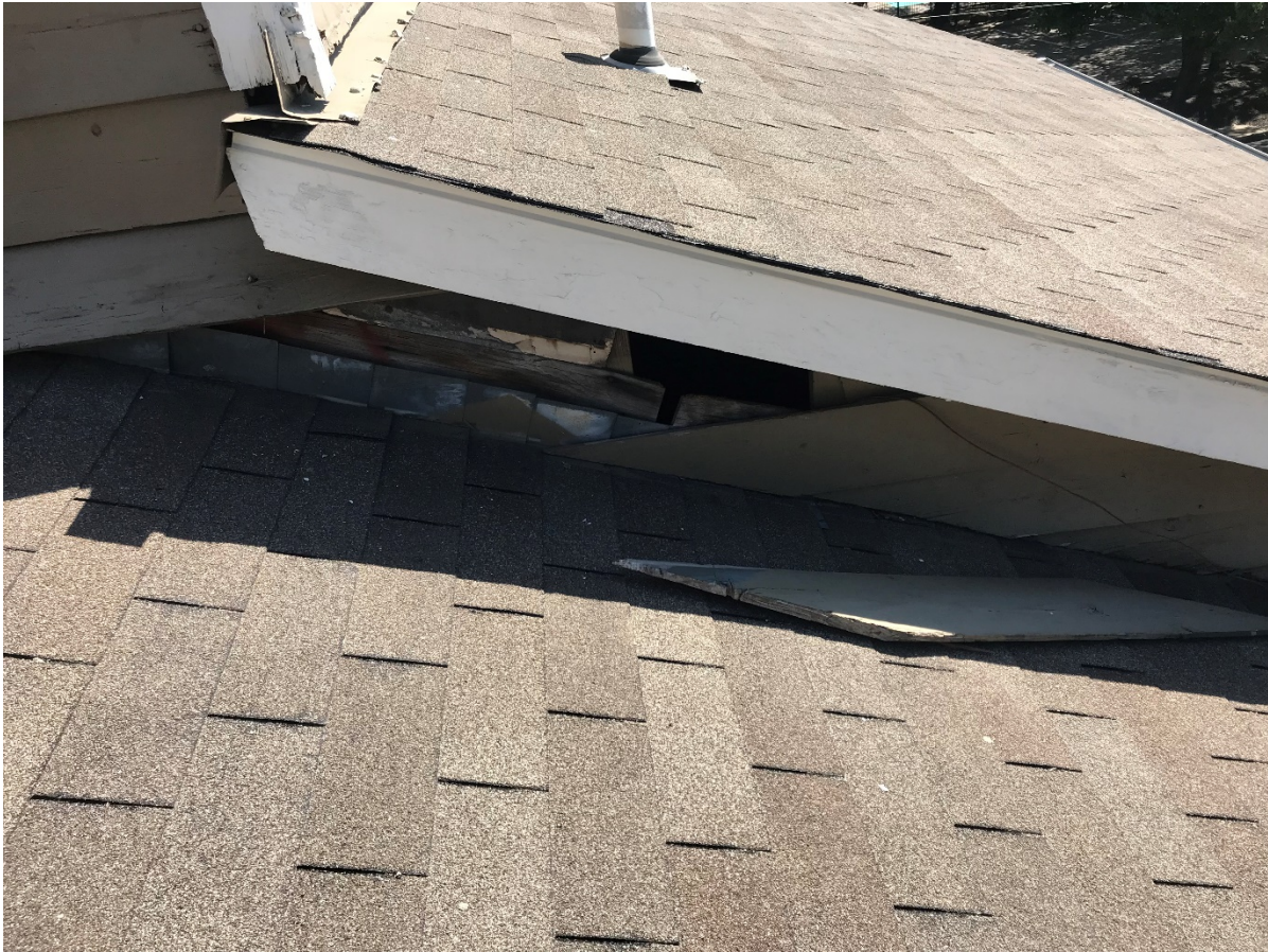
Repair missing or damage siding to replace step flashing
