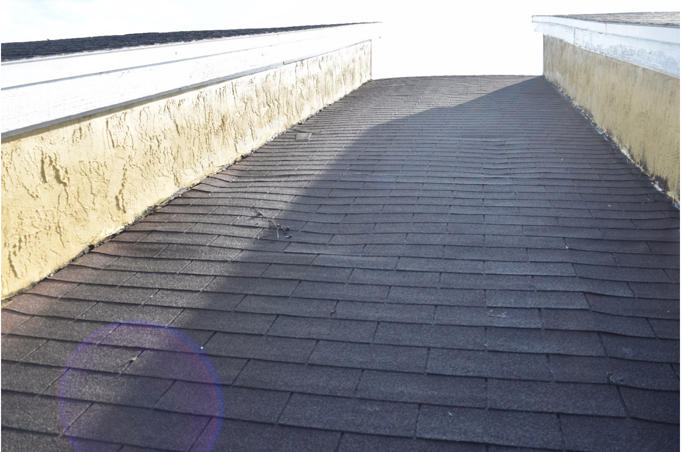
Remove stucco and install new step flashing and stucco weep screed 2 inches above shingles
