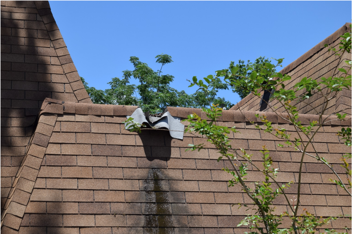
Fabricate new metal trough at all scuppers that drain onto shingle roofs
