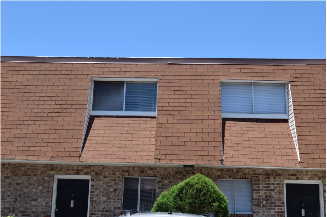
Shingles to be replaced or repaired
