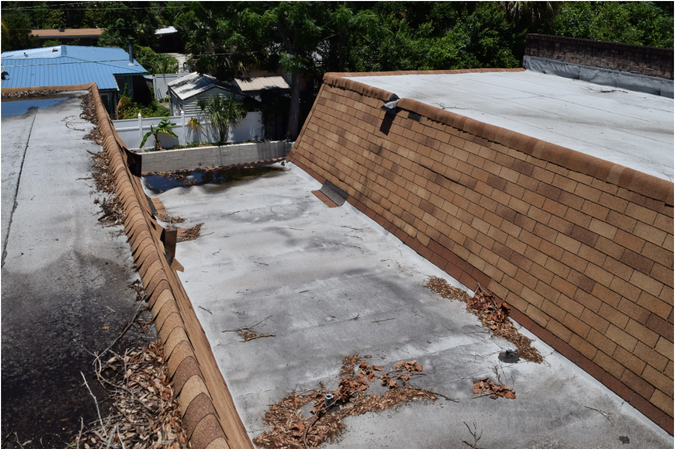
Fabricate new metal trough at all scuppers that drain onto shingle roofs
