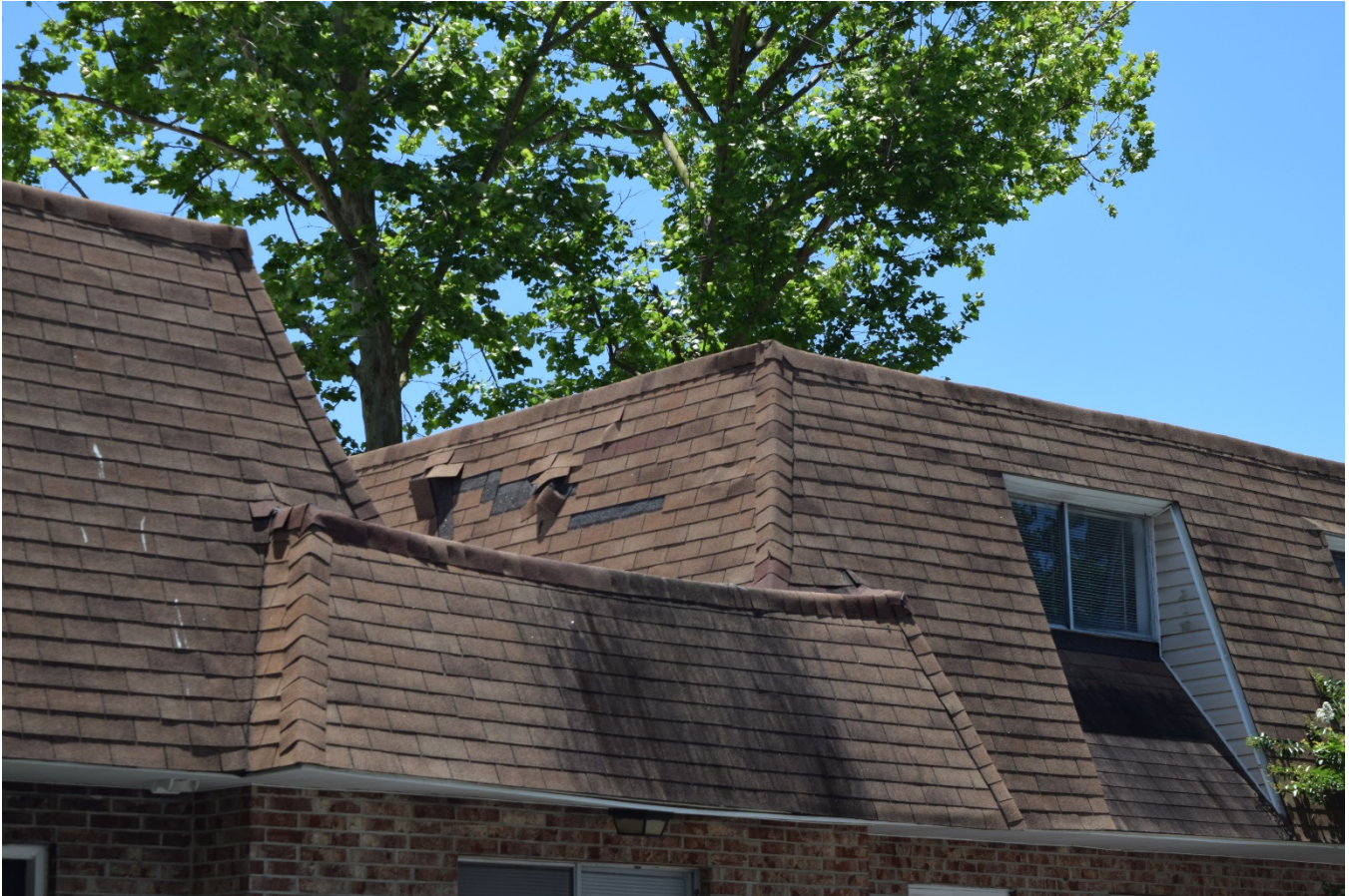
Shingles to be replaced or repaired
