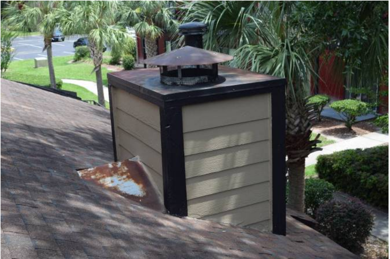
Remove siding to install new step-flashing and raise 1-1/2 to 2 inches above roof
